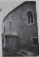
Fig. 182. A. Santa Rosa, Mexico. South wall of west chapel, showing round openings and right-hand pier.
